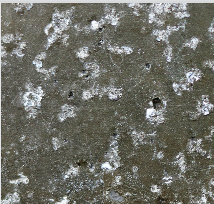
Details of surface corrosion
